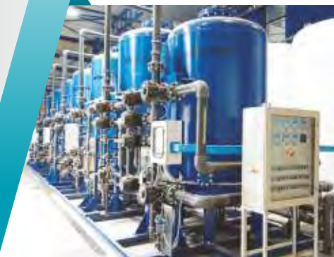
Demineralized Water Treatment Plant ( DM )
