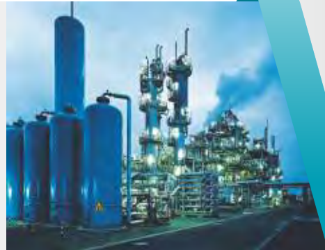
H2 / O2 Generation Gas Production Plant
